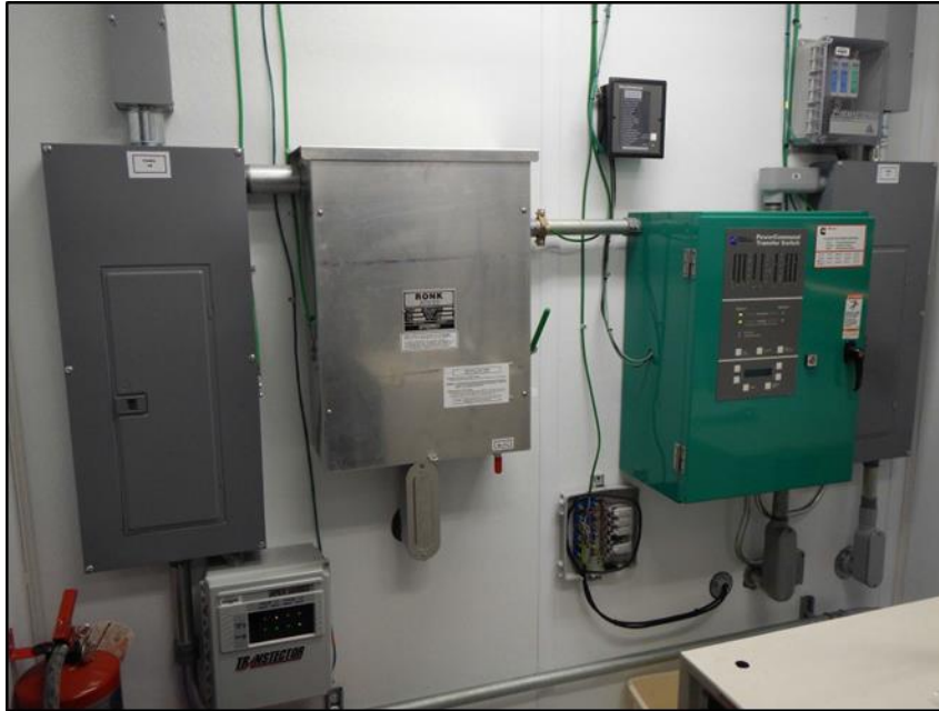
Figure 3c Power transfer panels
